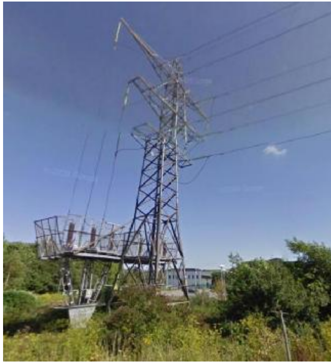
Photograph 2.1 - Typical Terminal Structure (located off the A473 north M4 Junction 35)
