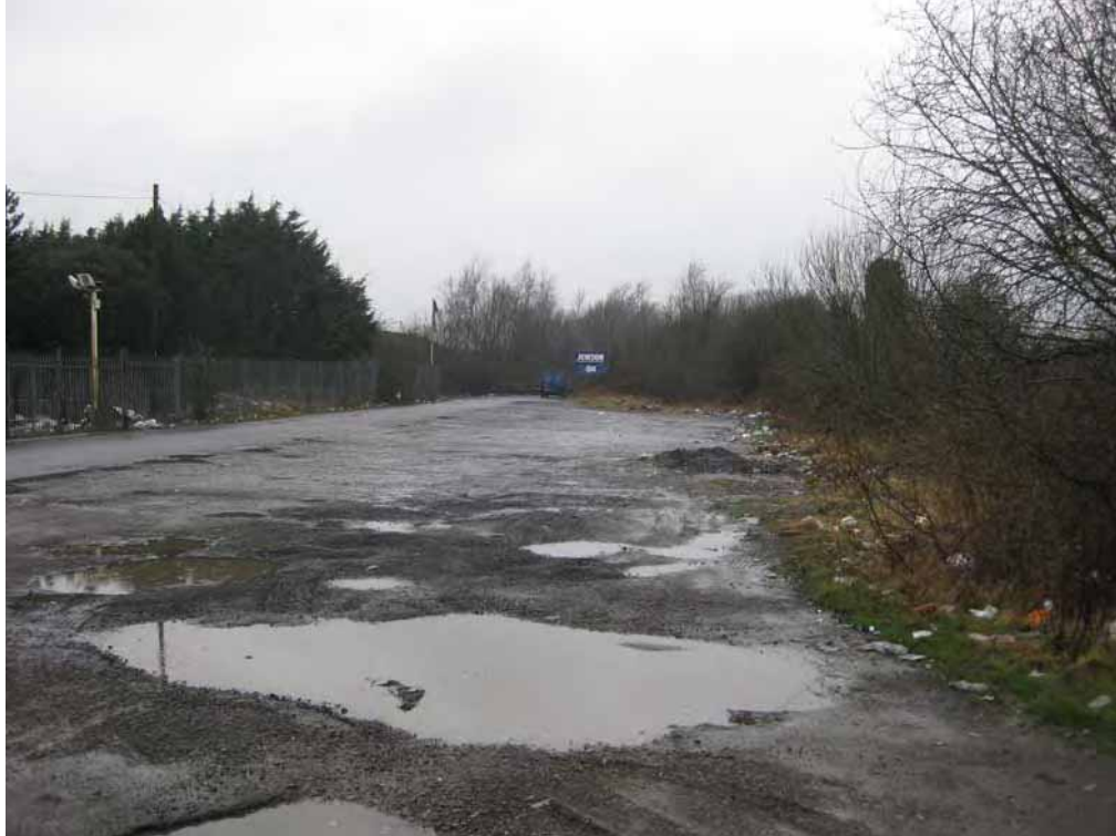
Plate 1 - Looking northeast, access is made directly from the B4181 Coity Road sign posted Jewson Builders Merchants.
